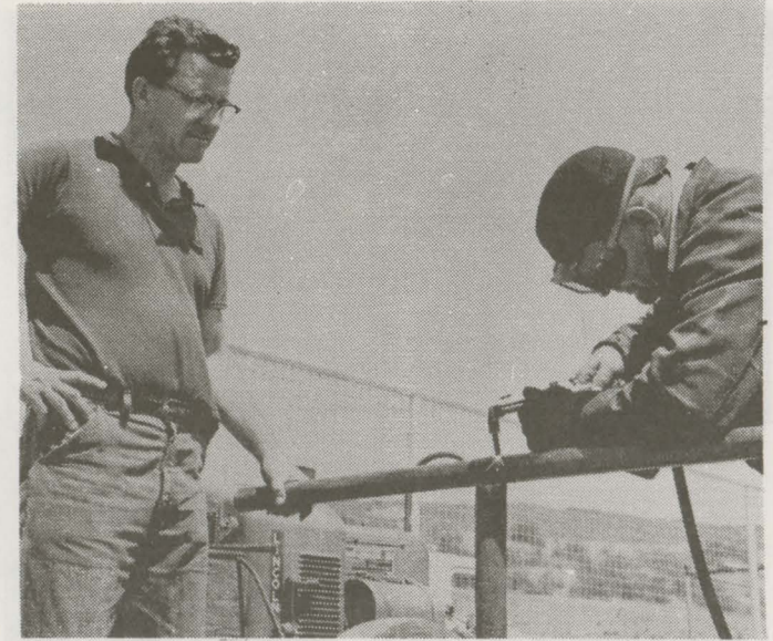
LARRY WILCOX LEFT ASSISTS KEN JERNEY IN PREPARING FOR THE BASEBALL SEASON WHICH STARTS THIS WEEK. THEY ARE MAKING A HANDRAIL FOR THE STAIRS LEADING TO THE FIELD. PHOTO BY JOHN GILROY
